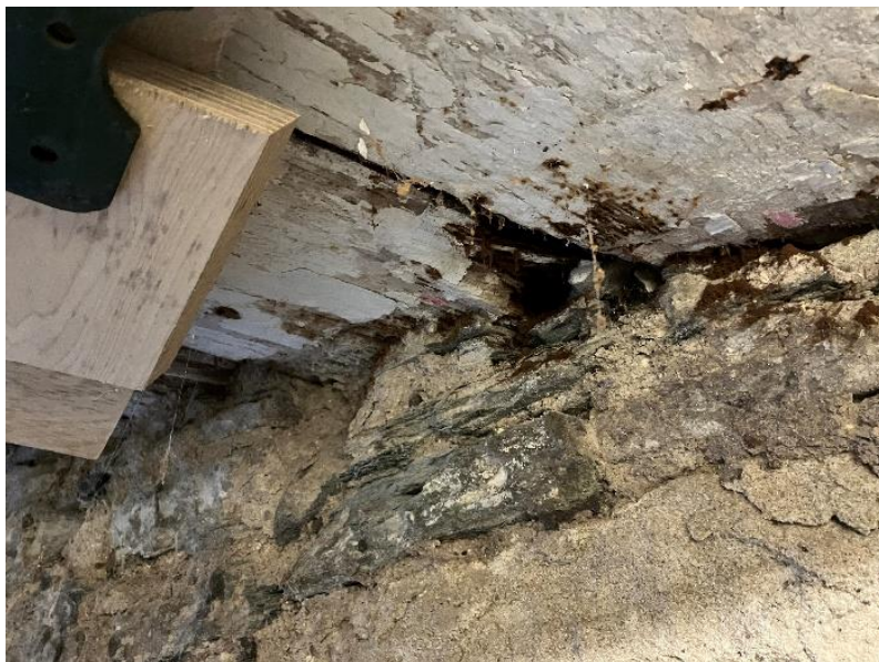
Fig 3. Timber lintols in B.12. This wood is spongy to the touch and decay has been principally at the ends of the timber, leaving the bearing very short.
