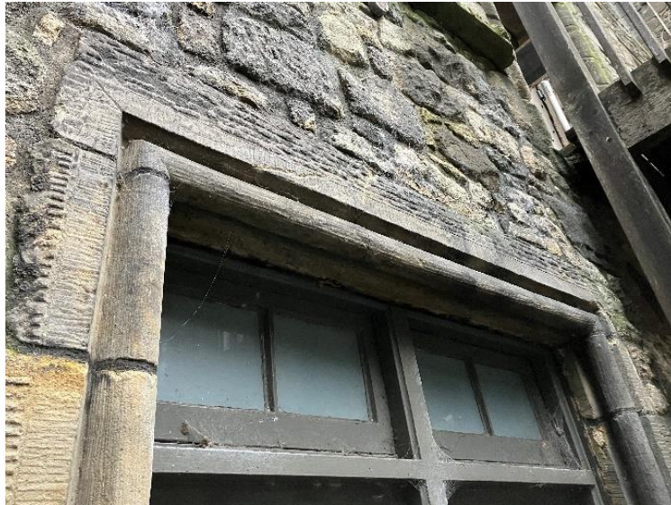
Fig 4. W:B.19. A vertical crack is visible near the centre of the stone lintol.
