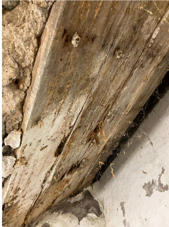
Fig 2. Image of the timber lintols in B.11. Decay is visible and the poor condition is evident. Photograph taken by Lewis Brunton.
