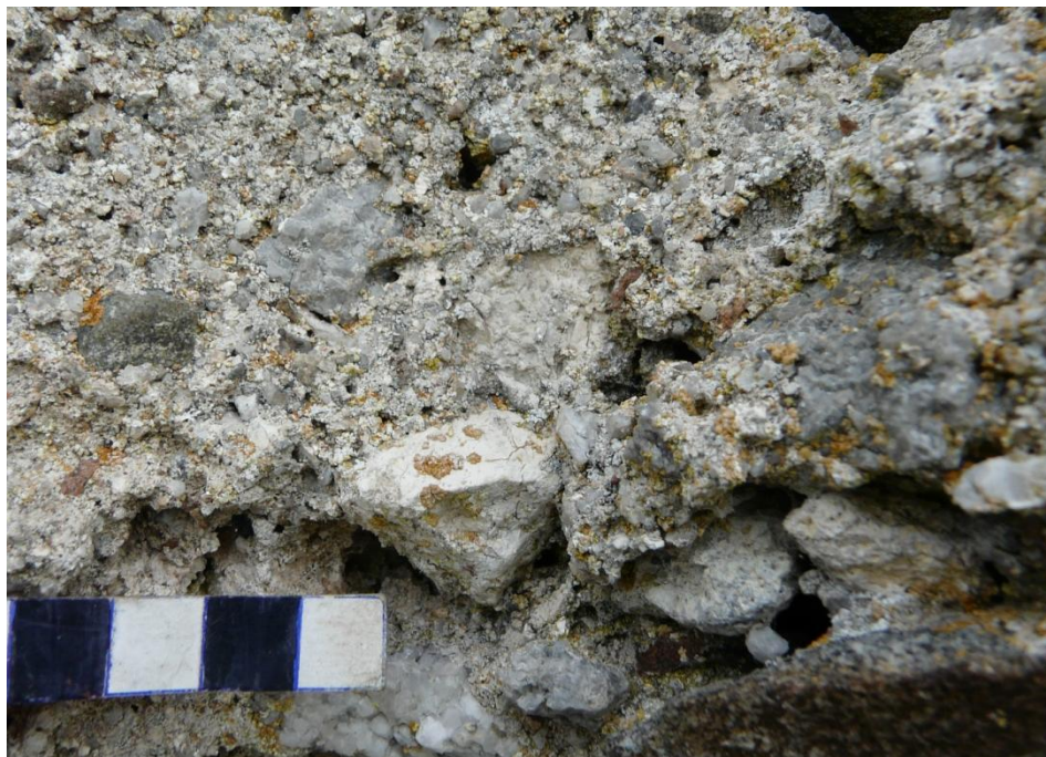
Figure 9 – Core mortar within the south-west wall of Castle Roy. Note high concentration of large angular probable heated limestone kiln-relicts. Scale 10mm; photograph M. Thacker.
