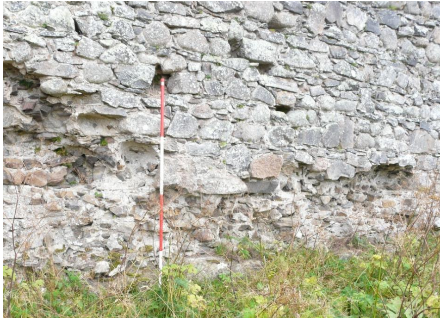
Figure 8 – Visible core rubble and constructional mortar exposed by missing face stone in external face of the north-west wall. Scale 500mm; photograph M. Thacker.
