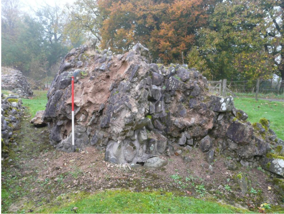
Figure 5 (above) – Context 1 from the south. Note area of degrading mortar to the right of the ranging rod and on the ground below. Scale 500mm; photograph M. Thacker.
