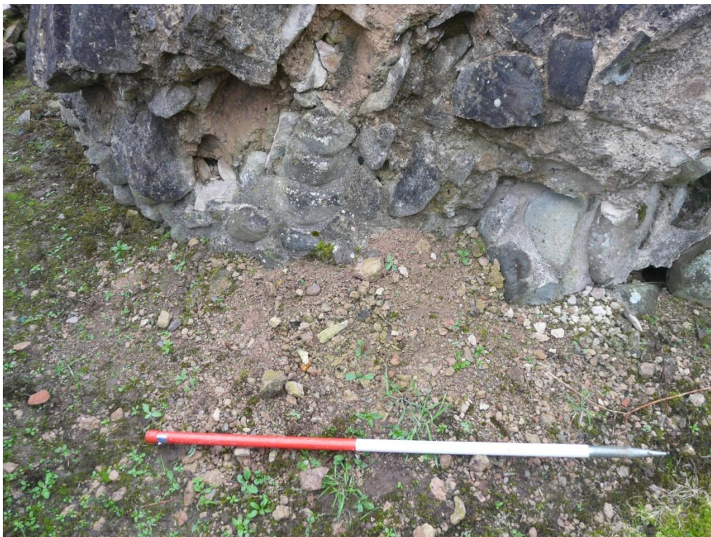
Figure 8 (above) – Degraded mortar at base of context 1. Scale 500mm; photograph M. Thacker.
