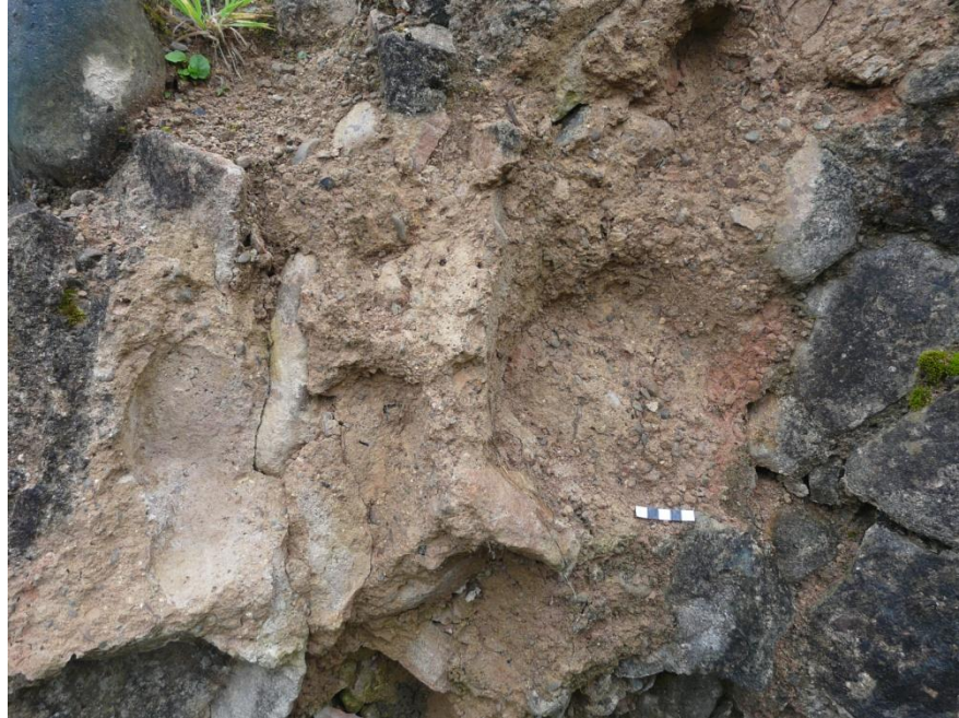
Figure 7 (above) – Degrading mortar in Context 1. Scale 10mm; photograph M. Thacker.
