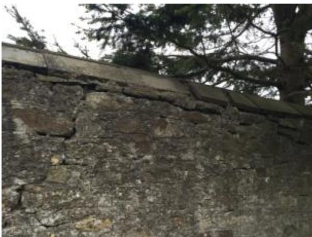
1: West Wall, East face Open joints to stonework
