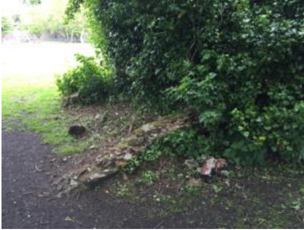
3: South Wall, close to path Partial collapse of wall
