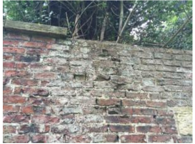
6: North Wall, South face Missing cope stones, defective brickwork and open mortar joints
