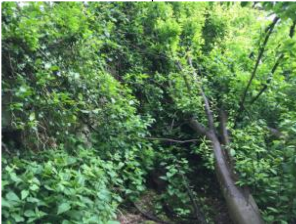
5: South Wall, South Face Fallen tree, possible damage to wall
