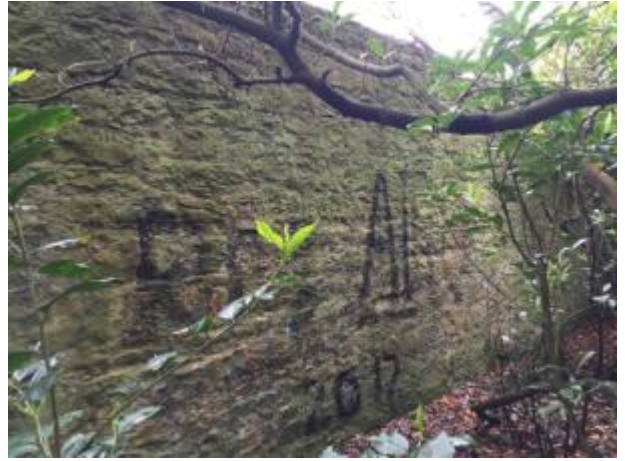
4: East wall, East face Graffiti to wall
