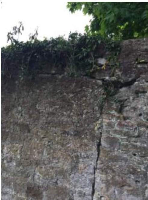
1: North Wall, North face Vertical crack to wall and open joints
