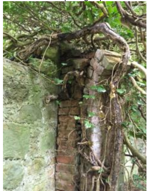
8: South Wall, South Face Excessive vegetation growth, defective brickwork
