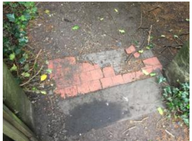
2: North/East corner, near opening Damage to floor tiles at opening
