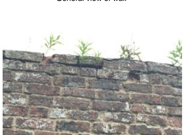
4: North Wall, South face Vegetation growth at high level
