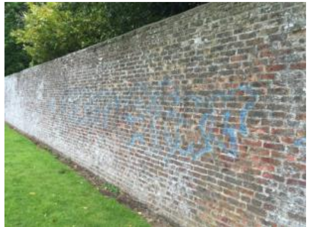
2: East wall, West face Graffiti to wall
