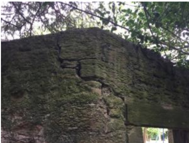
1: North/East corner, near opening Large open crack to stonework
