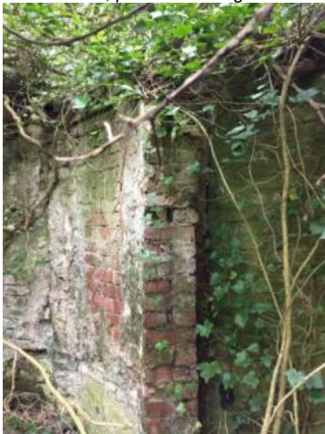
7: South Wall, South Face Excessive vegetation growth, defective brickwork
