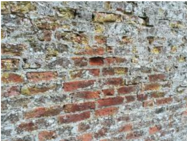
1: East wall, West face Defective brickwork, lichen growth to face of brickwork, open mortar joints
