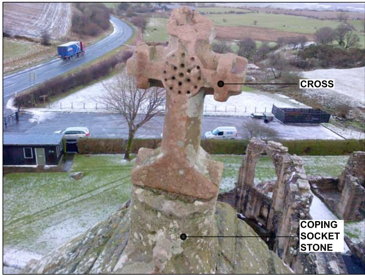
VIEW OF BELLCOTE CROSS PRIOR TO CROSS & COPING SOCKET STONE TEMPORARY REMOVAL DUE TO INSTABILITY.
