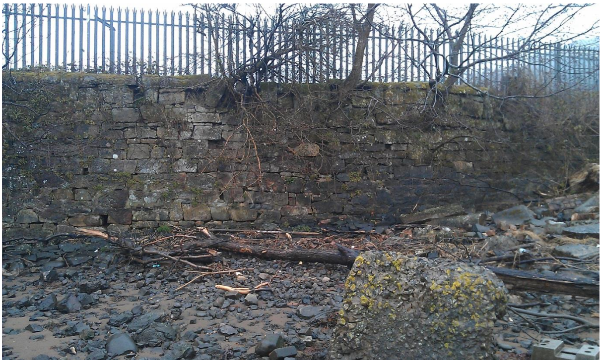
Vegetation damage occurring to the crest of the wall. Note storm debris at toe of the wall.
