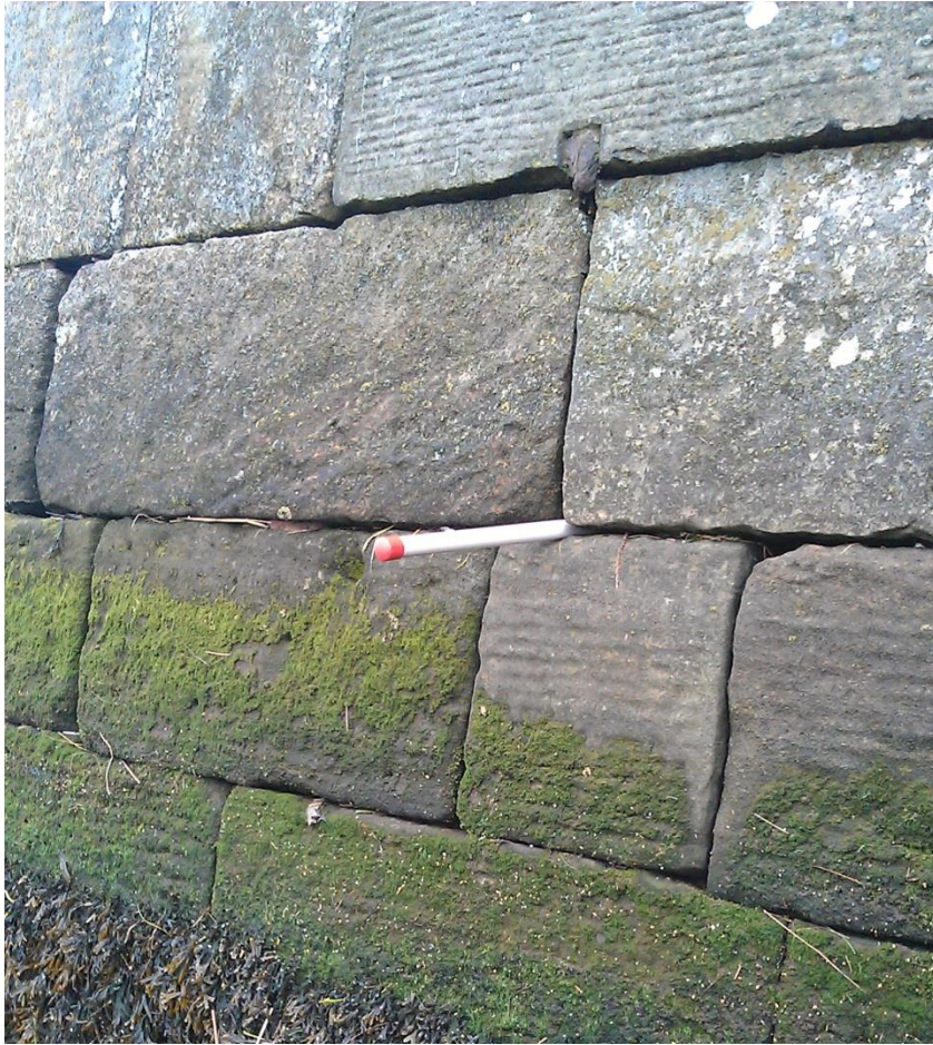
Voiding of 0.75 m behind facing blocks.
