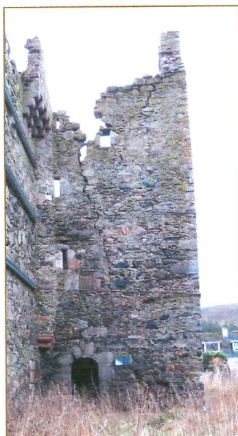
NORTH WALL OF TOWER EXTERNALLY; NOTE INSTABILITIES AT THE UPPER LEVEL
