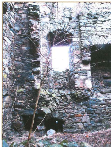
THREE PHOTOGRAPHS BELOW SHOW THE CONDITION OF THE EAST WALL INTERNALLY
