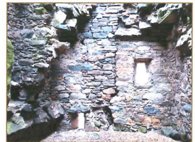
THE FLUE STARTS JUST ABOVE THE GROUND FLOOR VAULTS; NOTE LOOSE AND ERODED MASONRY AROUND.
