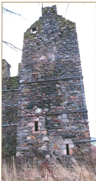
ELEVATION – NOTE FRAGILE AND ERODED MASONRY ALONG THE FLUE LINE AND AT THE WALLHEAD
