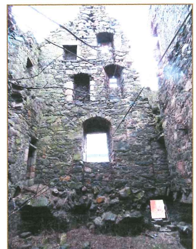
INTERNAL VIEW OF THE SOUTH WALL – NOTE UNDERCUT PIER OF THE TOP FLOOR WINDOW AND EROSION OF THE CHIMNEY
