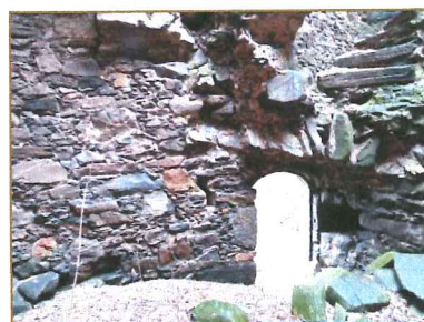
ERODED VAULT AND STAIR REMAINS ABOVE THE DOOR
