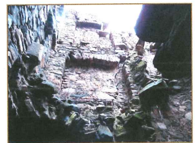
NORTH WALL OF TOWER INTERNALLY VIEW ON UPPER LEVELS SHOWING UNRESOLVED ARCHES AND PARTIALLY COLLAPSED PASSAGE
