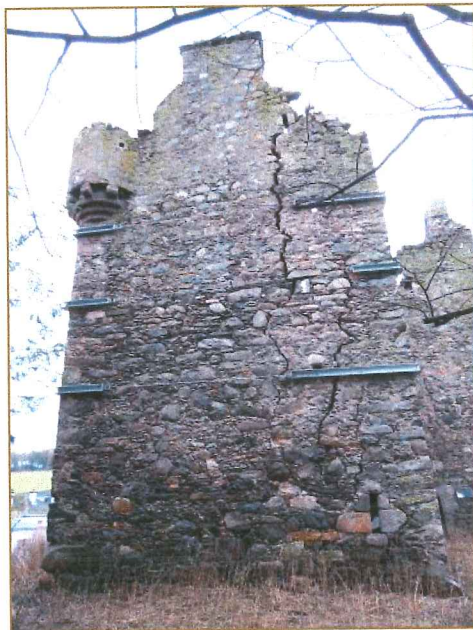
EXTERNAL FACE OF THE NORTH WALL VISIBLE LARGE CRACKS
