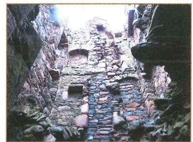
VIEW ON UPPER PARTS OF THE WALL. NOTE LINE OF THE FLUE TWICE CHANGING IN DIRECTION. THE MAIN CRACK FOLLOWS THIS LINE. ALSO, NOTE THE ERODED AND OVERHANGING STONES AROUND THE FLUE AT THE TOP FLOOR AND SPLIT ARCH OF THE RECESS
