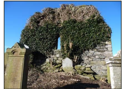
OVERGROWN EAST GABLE
