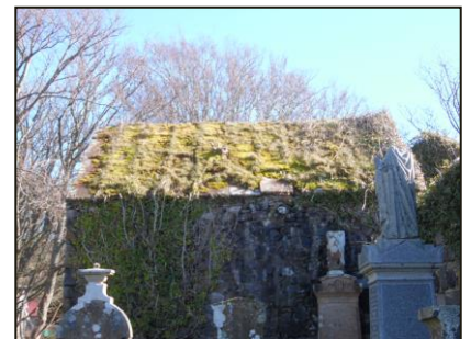
NORTH AISLE COVERED WITH VEGETATION, VISIBLE ORIGINAL ROOFING SLABS
