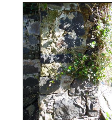
SOUTH WALL AT DOOR – NOTE EXTERNAL SECTION OF WALL LIFTED AND PUSHED OUT BY IVY
