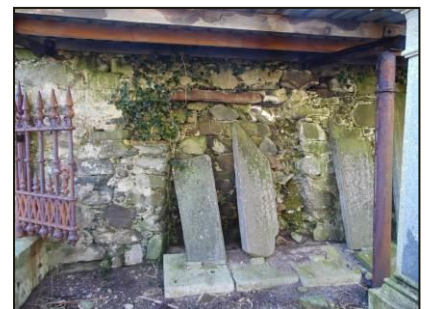
UNSUPPORTED ORIGINAL LINTEL
