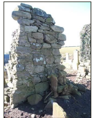
SOUTH WALL STUB – NOTE LARGE TREE ROOT AT THE BASE
