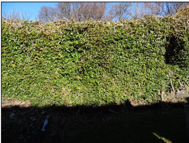
NORTH WALL INTERNALLY - HEAVY IVY GROWTH
