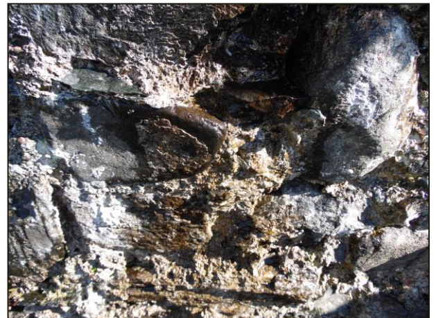
WATER RUNNING ON THE WALL FACE UNDER IVY
