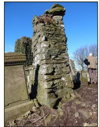
“STUB” – PUSHED BY TREE ROOT FROM INSIDE AND WITH VOID AT FOUNDATION LEVEL
