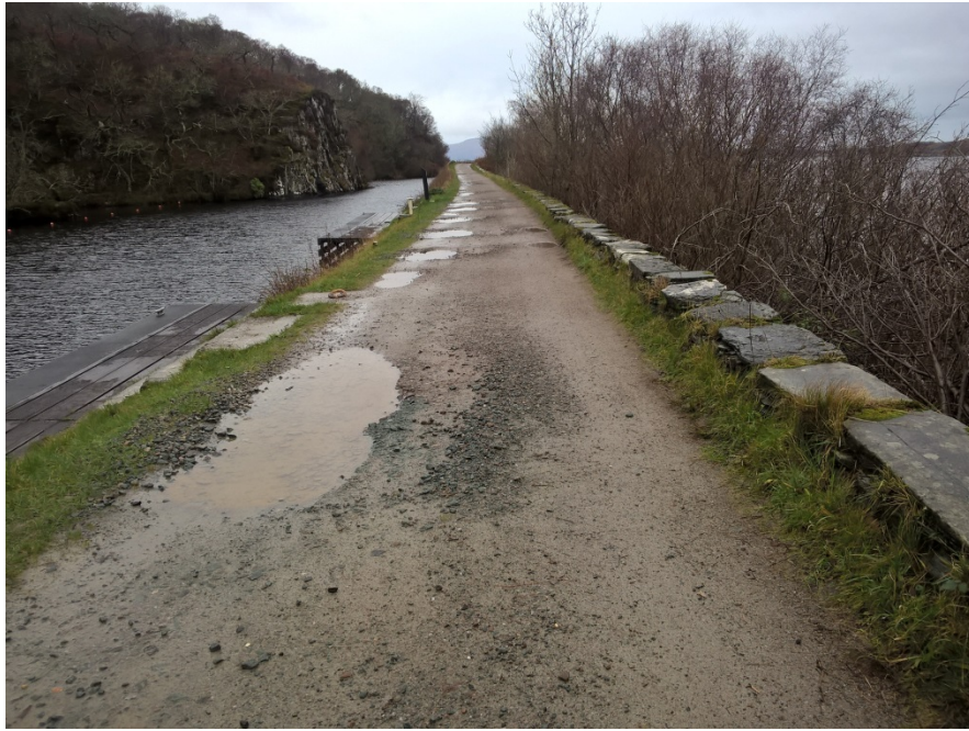
Typical existing soft towpath condition mooring can be seen on the left
