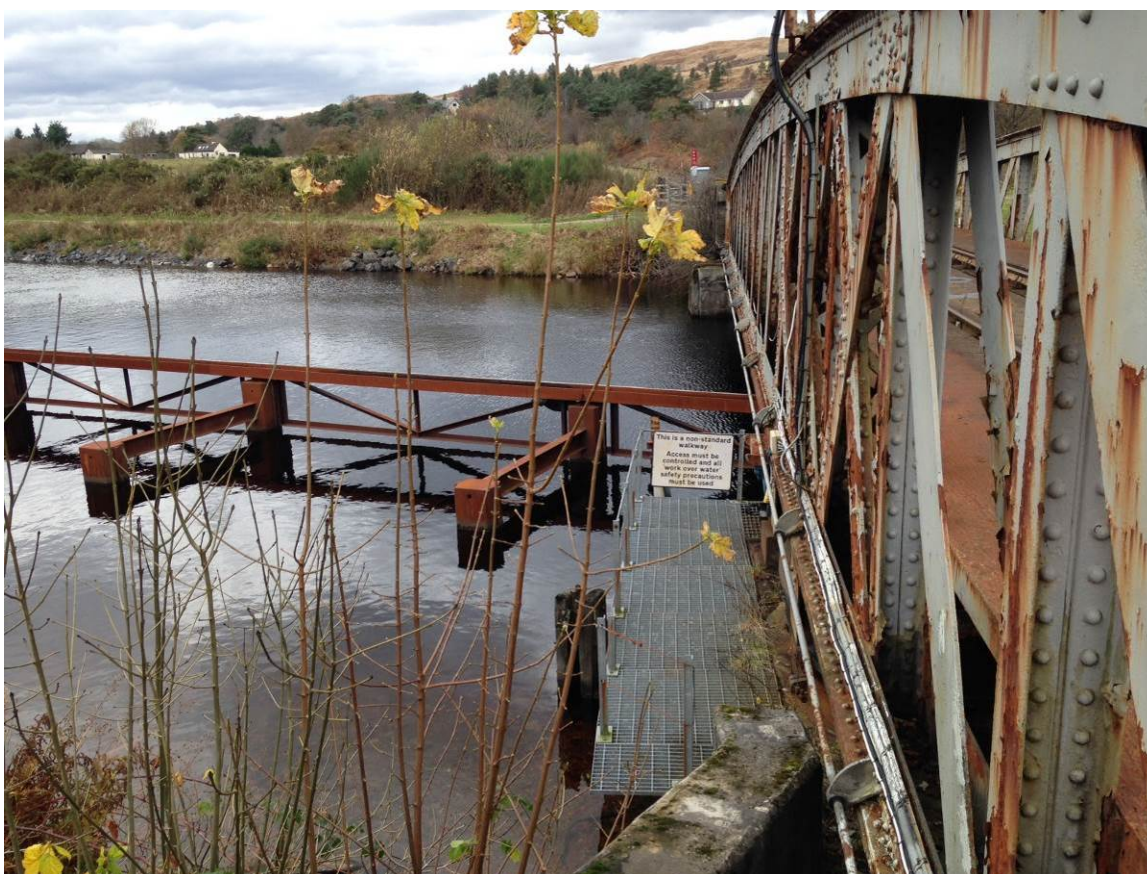
Photograph 3: area to SW where bridge swings when in an 'open' position
