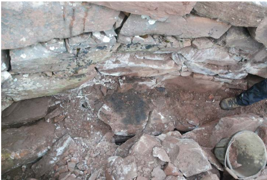
Figure 2: Burning on the scarcement ledge encountered during the 2012 conservation works.
