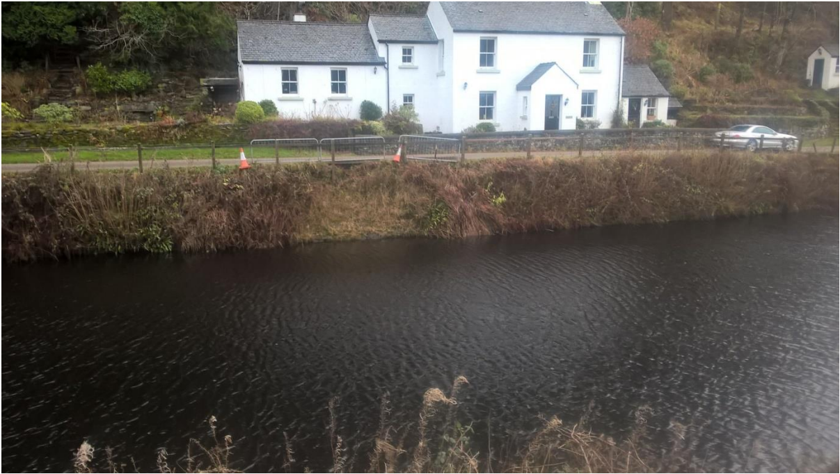
View of Area of Subsidence
