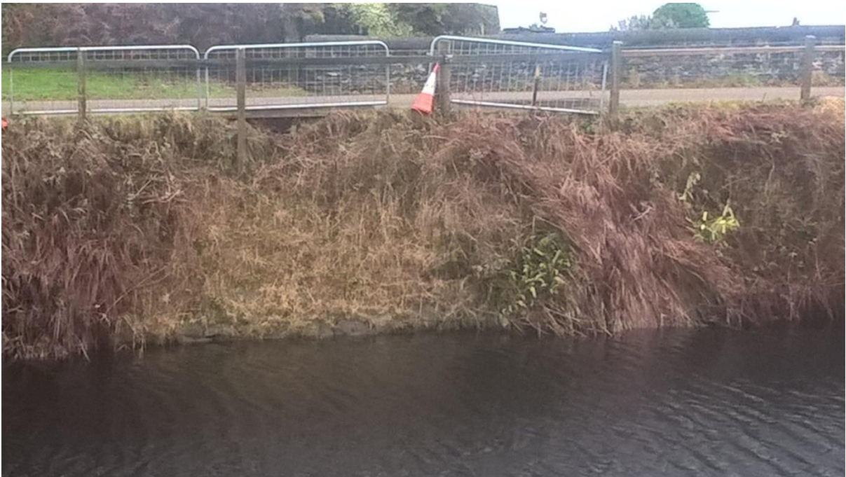
View of Area of Subsidence
