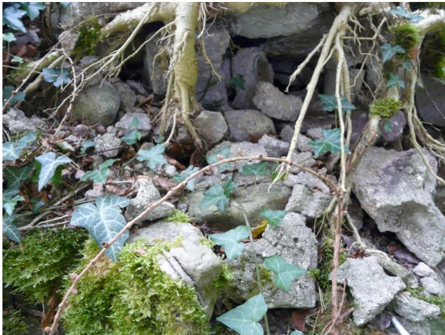
Figure 2 (above) – Kinclaven castle; wallhead of south-east wall includes contexts with quantities of detached core mortar fragments. No Scale; photograph M. Thacker.
