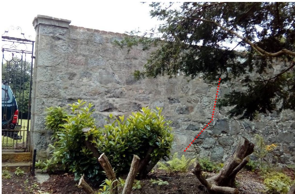
Illus 25 S wall W of central gate. Red line indicates break in construction
