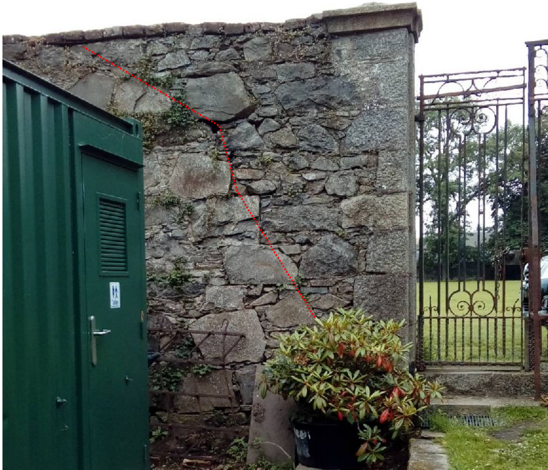
Illus 24 S wall E of central gate. Red line indicates break in construction
