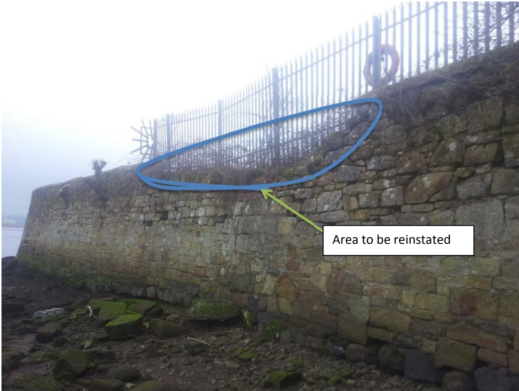
Picture 2 - Extent of reinstatement required
