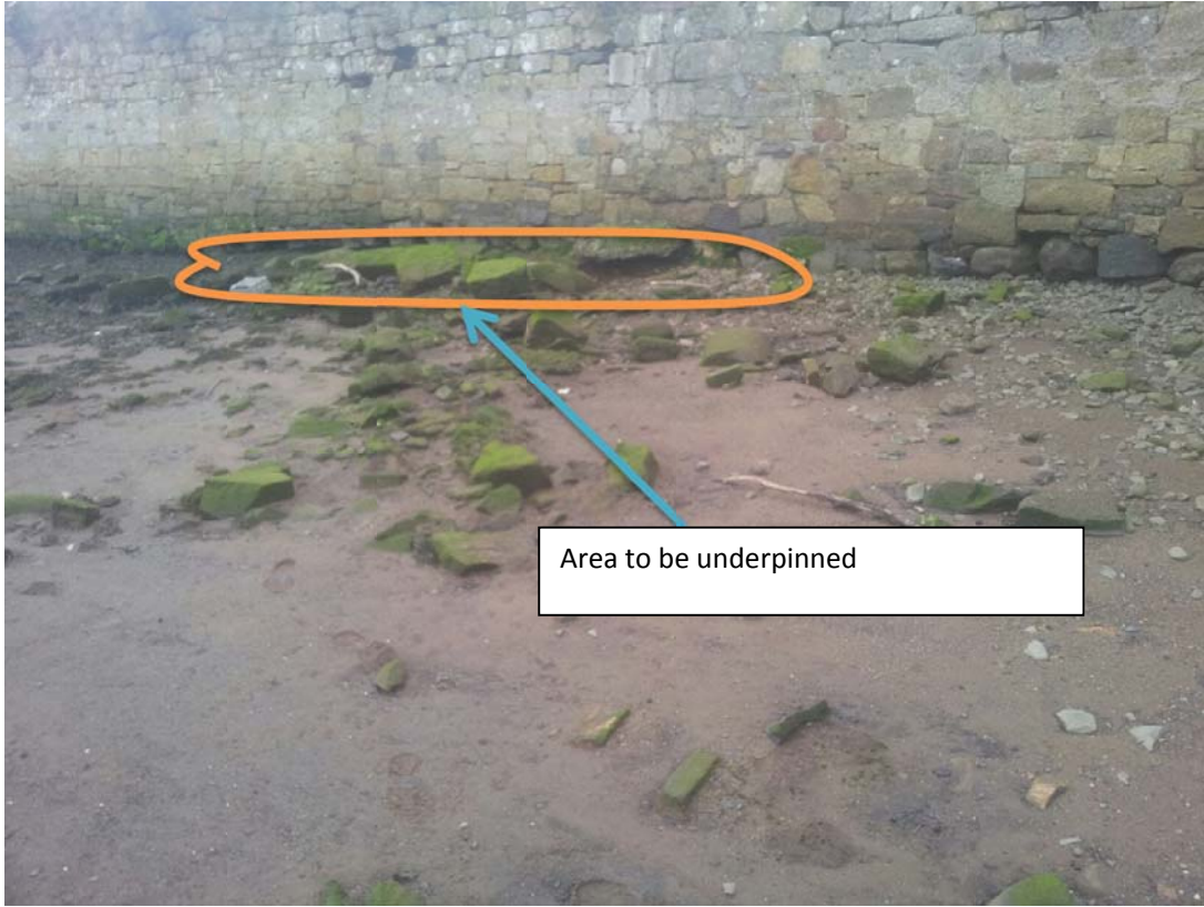
Picture 1 – Extent of underpinning required
