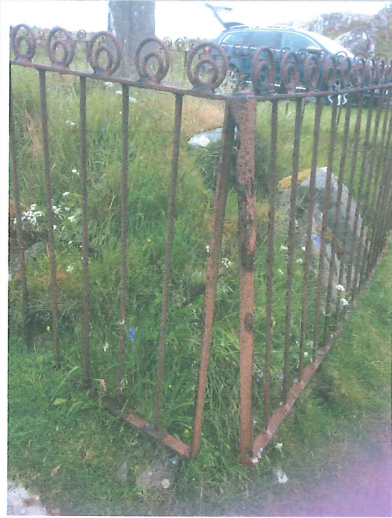
Large stone fallen and rolled-out into railings, causing damage to railings.
