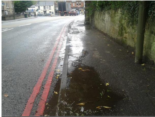
Slateford aqueduct canal leakage at footpath and road level
