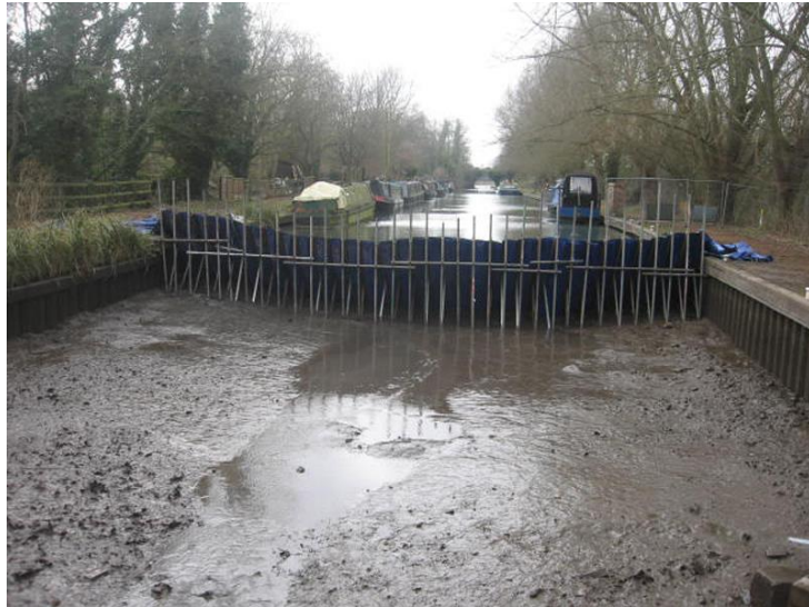
Fabric dam deployed in canal channel
