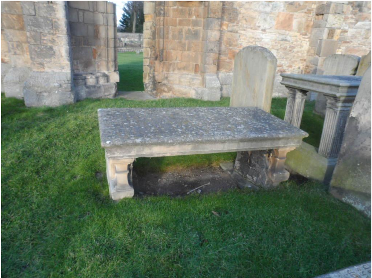
Typical table tomb showing dry soil underneath where vermin dig (revealing bones), and weeds grow)
