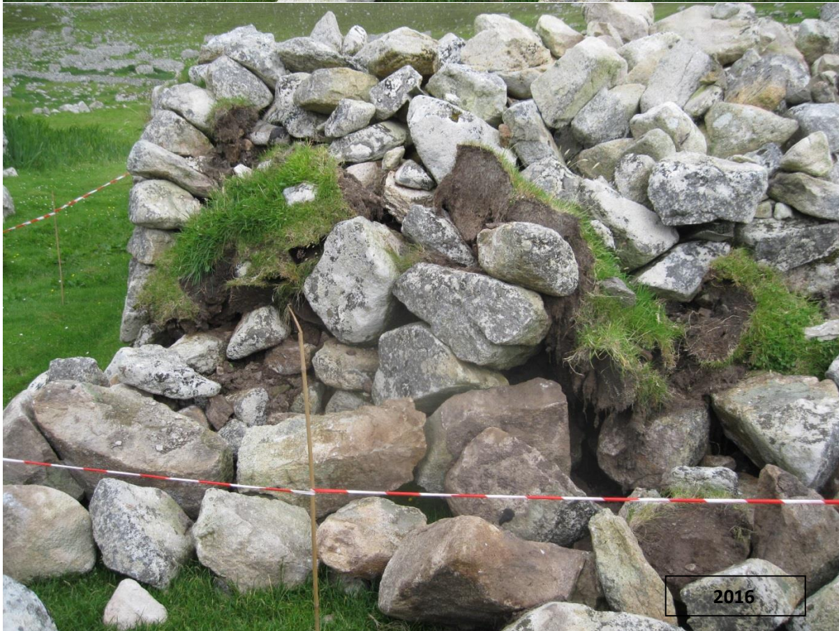
Figure 9 Detail of collapsed stonework of south gable of blackhouse H in July 2016
