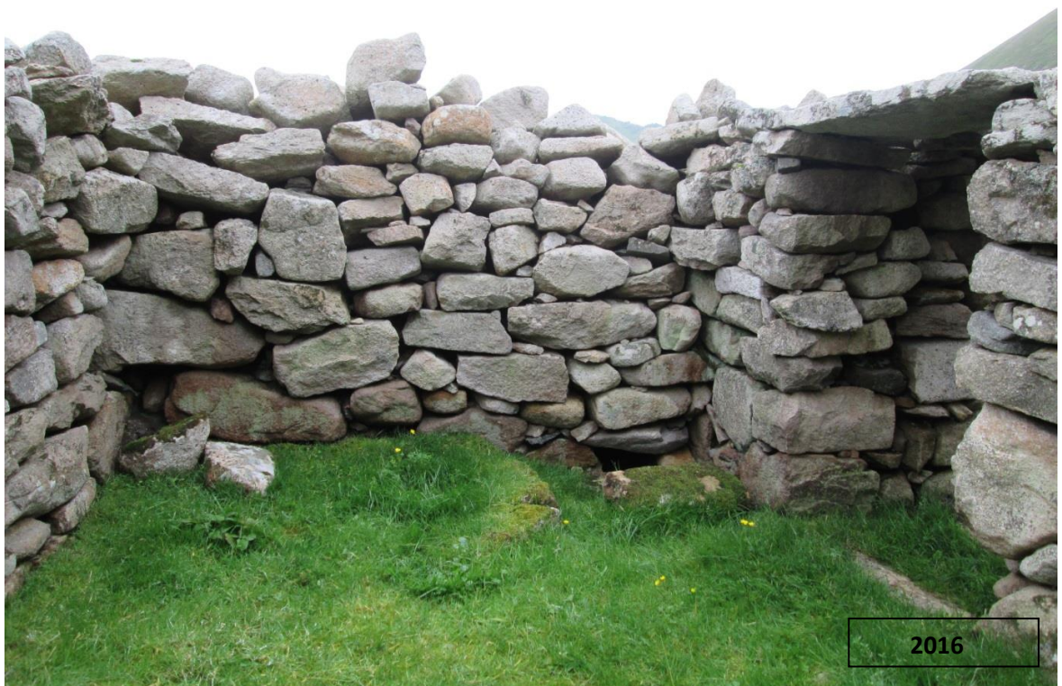
Figure 8 Blackhouse H interior view of south gable as surviving in 2008 and August 2016
