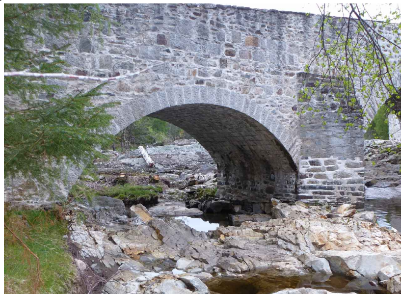
Photo showing current bank condition (NTS)
