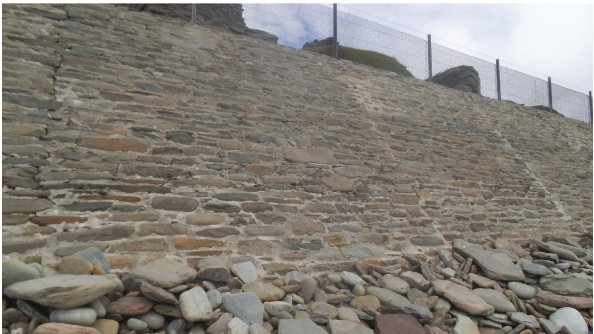
10. A typical mid-wall section showing the regular bay/failure/expansion pattern in addition to the general decay of the previous pointing
