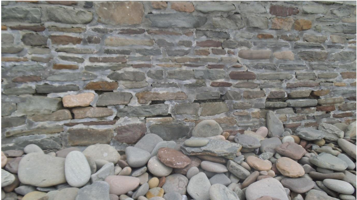
7. Voids being formed at wall base behind hard cement pointing, typical to whole wall
