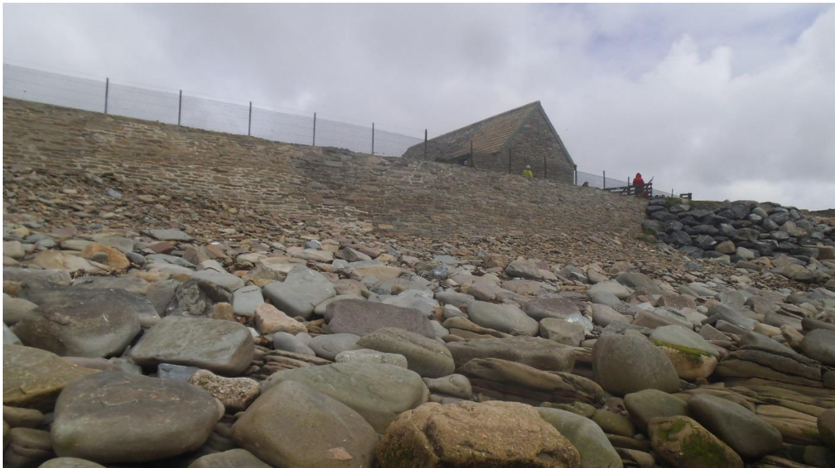
2. Wall showing pointing patches from previous works
