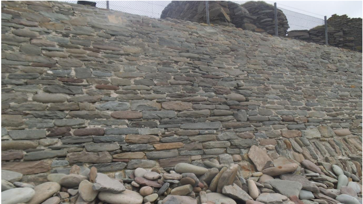
9. Much previous patch mortar, voids evident where hard pointing has fallen away
