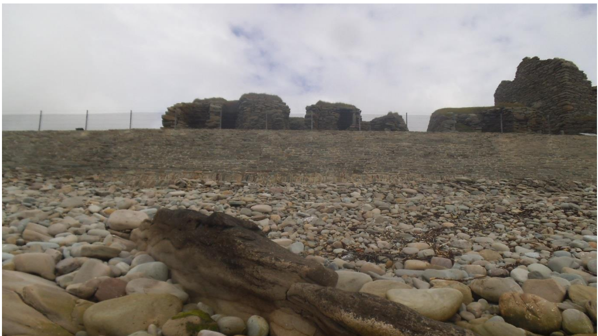
4. Patches of previous repair, dark spots where mortar is missing, regular decay lines relate to wall construction bays
