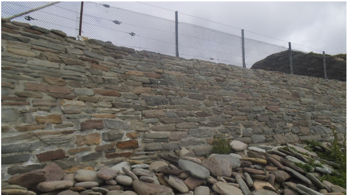
8. Hard pointing losing hold on stones, voids forming behind, wall top stones becoming loose/dislodged
