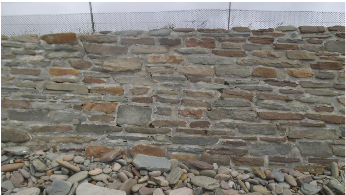
6. Voids behind strong cement mortar in western region of wall
