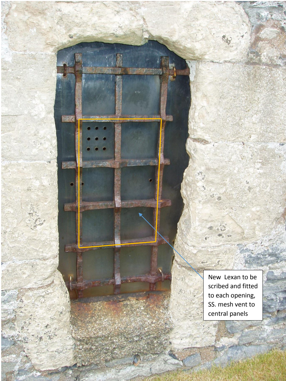
Typical yett fenestration. New Lexan to be fitted to each opening. Stainless steel bar frame secured with SS. 'P' clips to Lexan to carry SS. net to form vent to central panels.
