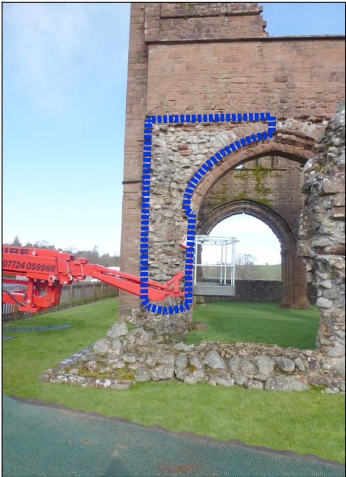
Core to South Aisle wall to be consolidated. Adjacent decayed dressed sandstone to be brushed back and repointed.
