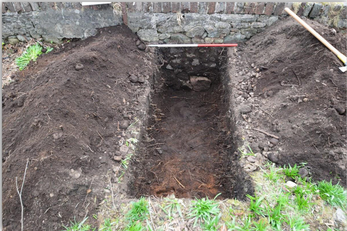
Illus 5 View of completed Trial-pit 2 prior to backfilling. Note gradual change from reddish-brown natural at top to darker more organic natural along wall.
