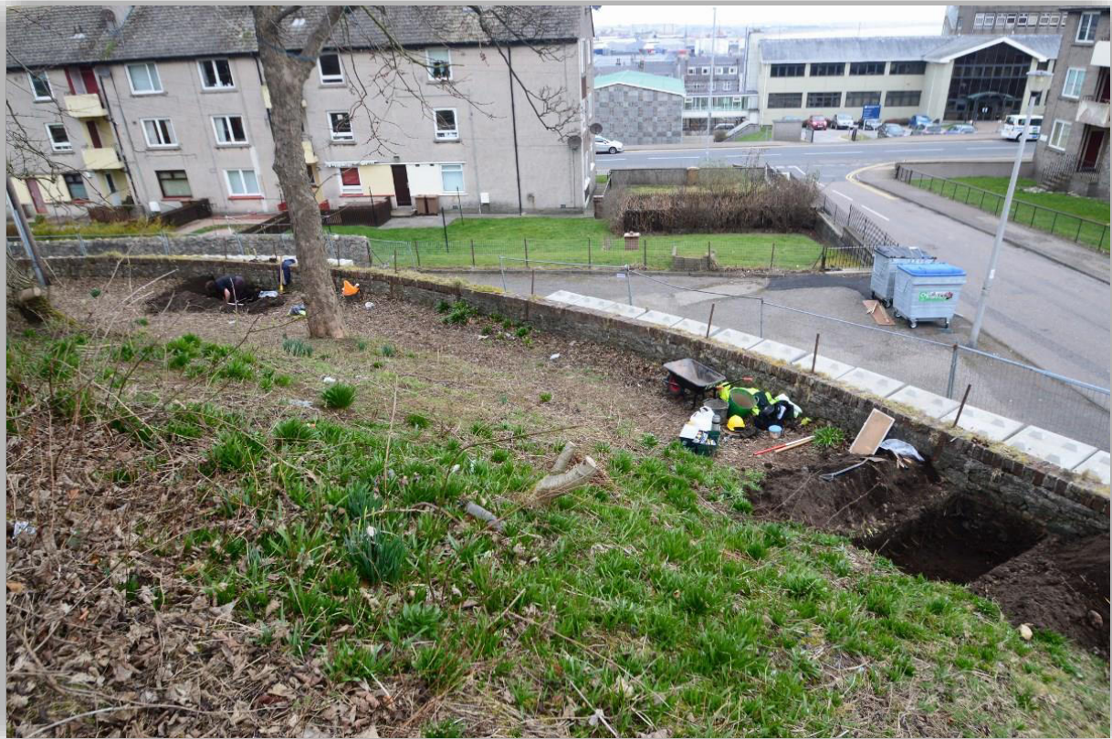
Illus 4 General view of trial-pit locations along the retaining wall for Balnagask Motte with TP1 (left) and TP2 (right); facing N
