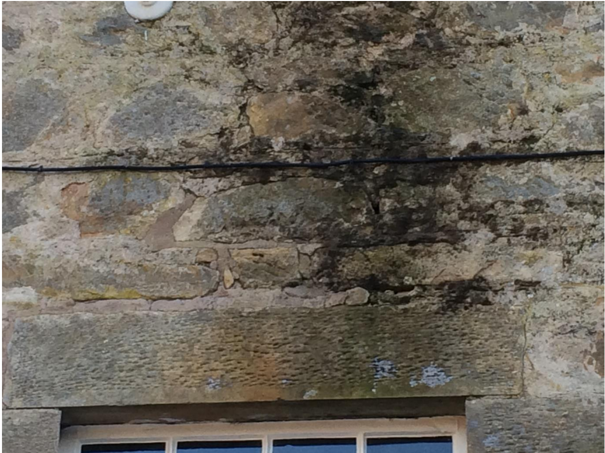
Water staining to the external kiln wall
