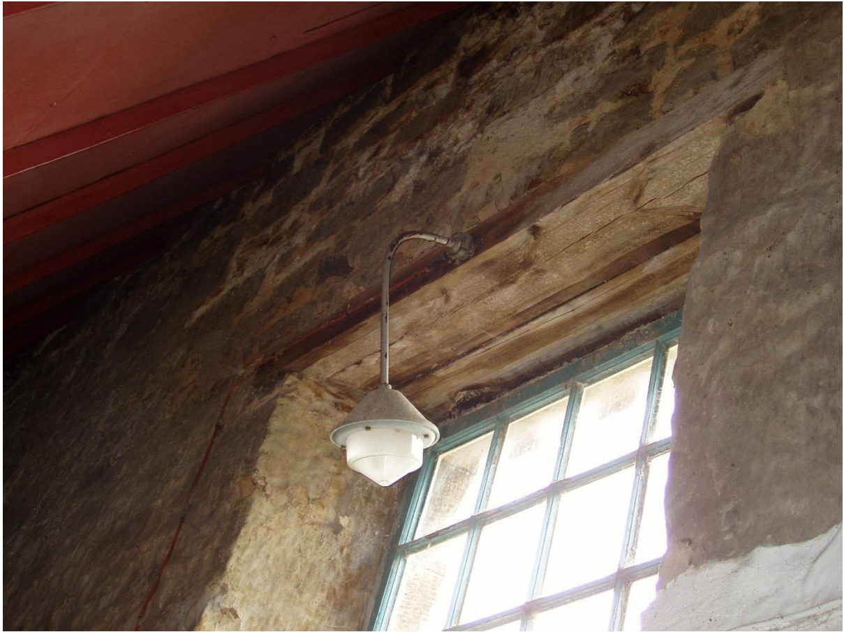
Lintel of large kiln window (note old fruiting body). Break out rotten lintel and reinstate with treated timber coated with Boron, locally rebuild masonry and slaister to match as required.
