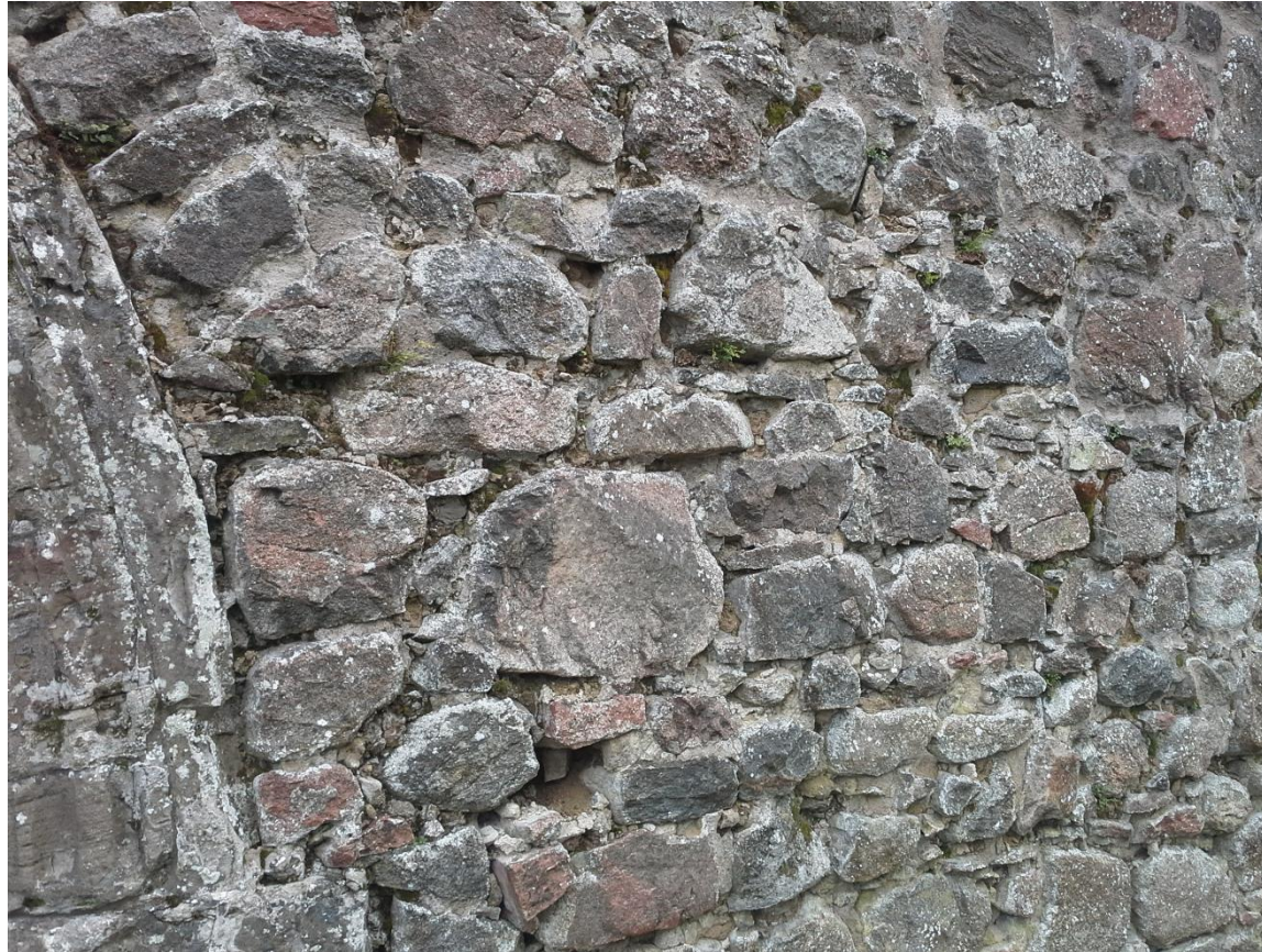
Photo 6: Areas of eroded pointing on elevations
