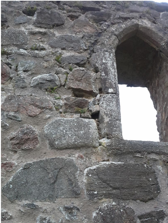
Photo 4: Deterioration of pointing around window on east gable
