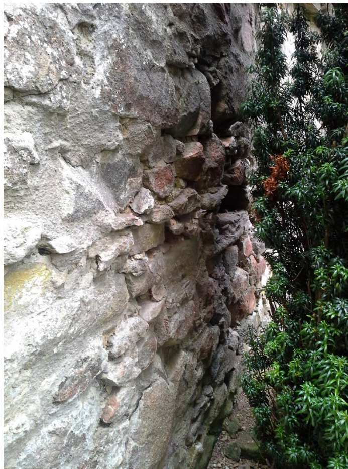
Photo 2: Eroded pointing behind yew tree
