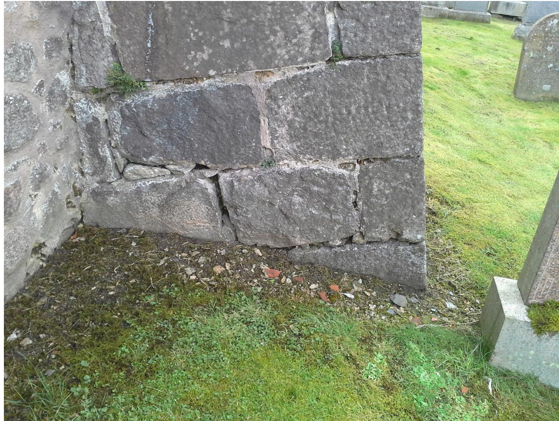
Photo 5: Deteriorated mortar in joints of granite buttress
