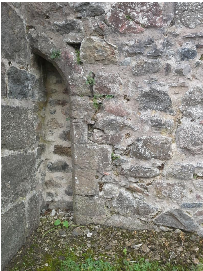
Photo 1: Deteriorated recent attempts of re-pointing using cement
