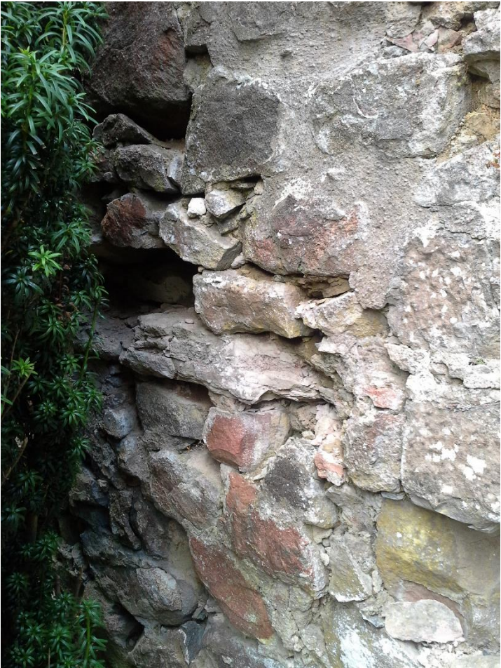
Photo 3: Large area of eroded pointing behind yew tree
