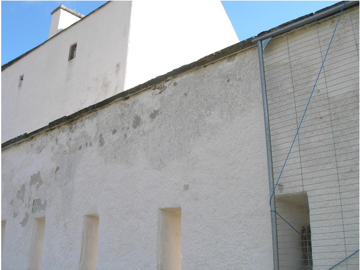
The failing harl to the north wall before its removal in 2011, note delaminating old copes.
