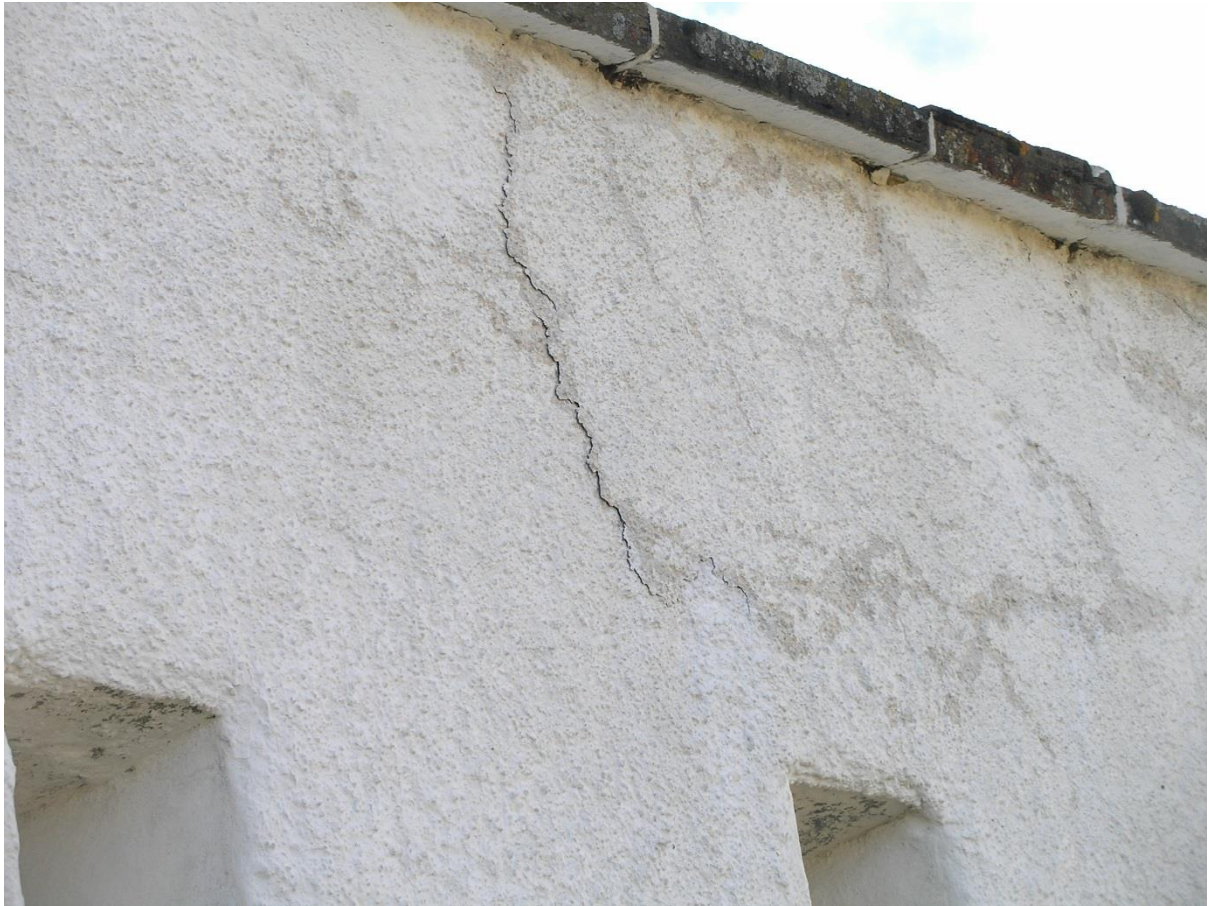
The failing harl to the north wall before its removal in 2011, note delaminating old copes.
