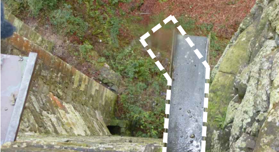
Photo 11 - Spout needs to be re-directed away from wall.
