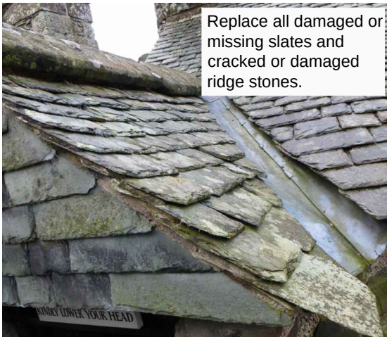
Photo 6 - Loose slate at verge/eaves.
