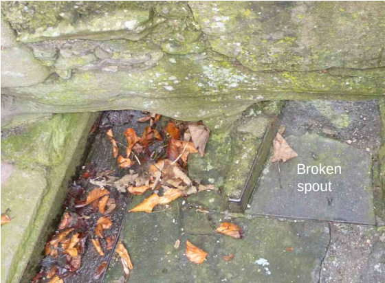
Photo 12 - Renew broken steel spout and insert new steel spout insert to exist. stone spout to throw water away from walls.
