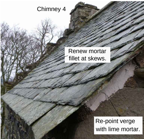
Photo 4 - Loose slate at verge/eaves.
