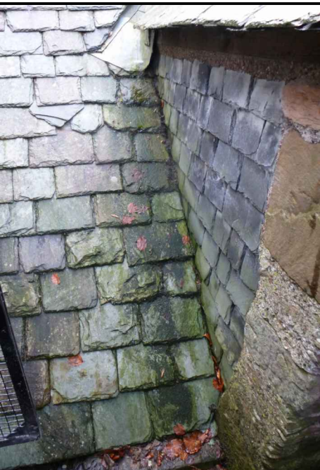
Photo 10 - Secret lead gutter blocked, Clean out.
