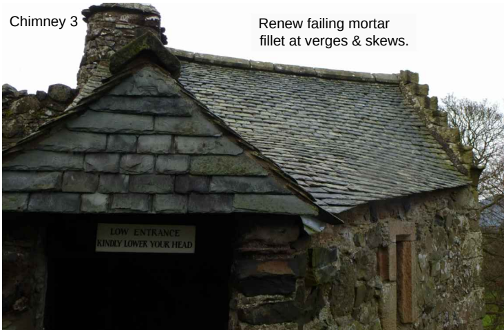
Photo 5 - Loose slate at verge/eaves.
