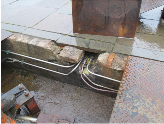
Damaged Brickwork at Ram Pits
