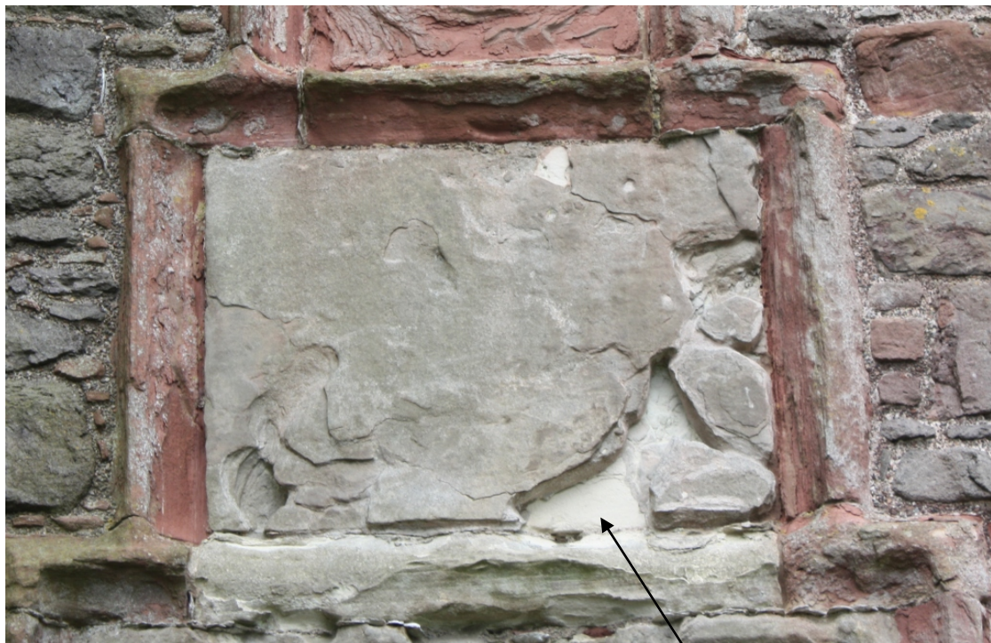
Middle panel with area of recent loss
