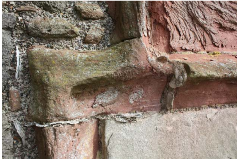
Eroded moulding with protruding shell pinning
