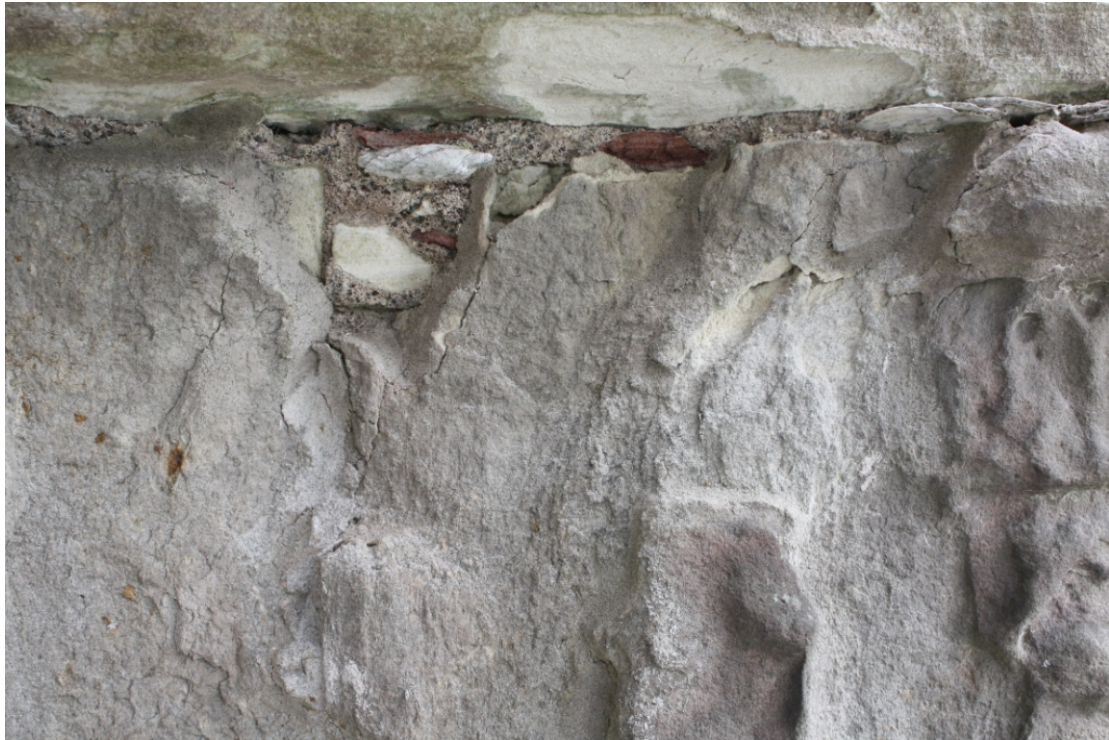
Failing resin repairs and surface delamination at centre of top edge
