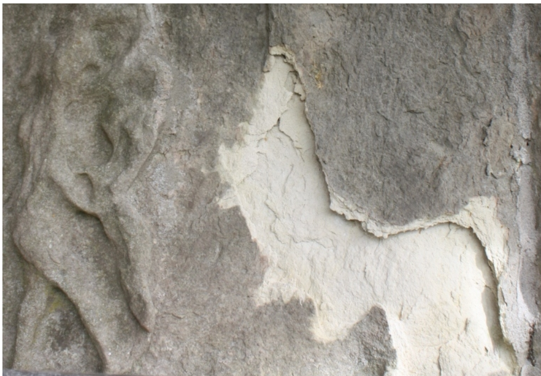
Area of recent loss from surface delamination with exposed disaggregated substrate
