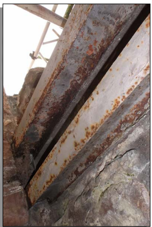
Photo of corroded beams to be replaced
