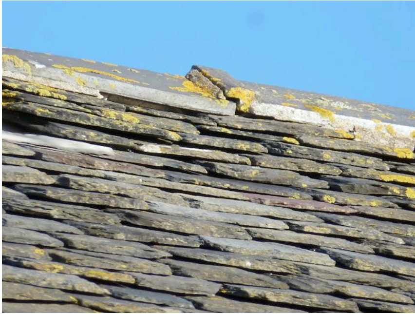
Photograph 7: Roof and ridge on visitor centre showing gaps in mortar and underneath slates.
