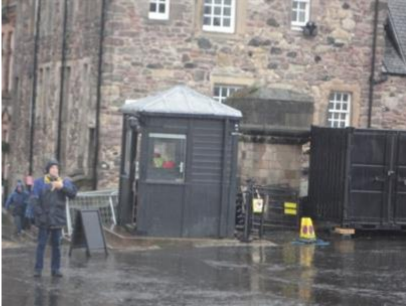
Fig.8 The present Bottom Box. The lower section has been overclad with ply because of rot in the original timber boarding and floor.
