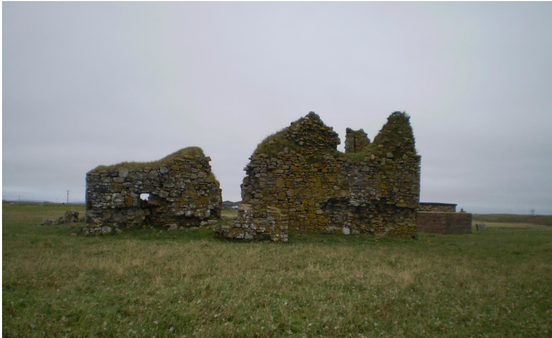
Figure 1 – Castle Borve, Benbecula showing large areas of masonry core at ground level.
