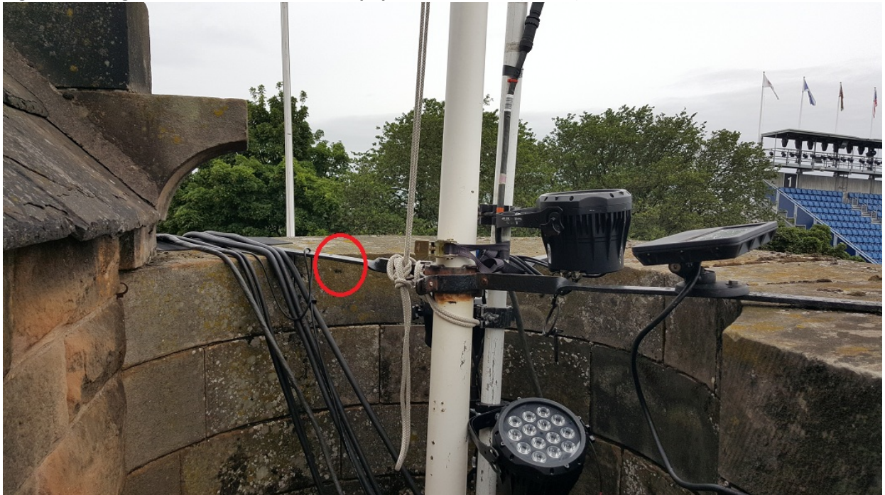
Fig. 5 Edinburgh Castle Gatehouse roof equipment location (North)
