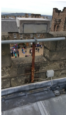
Fig. 23 Edinburgh Castle Palace roof west: access point and point to multipoint location, wiring will be concealed below existing lead flashings
