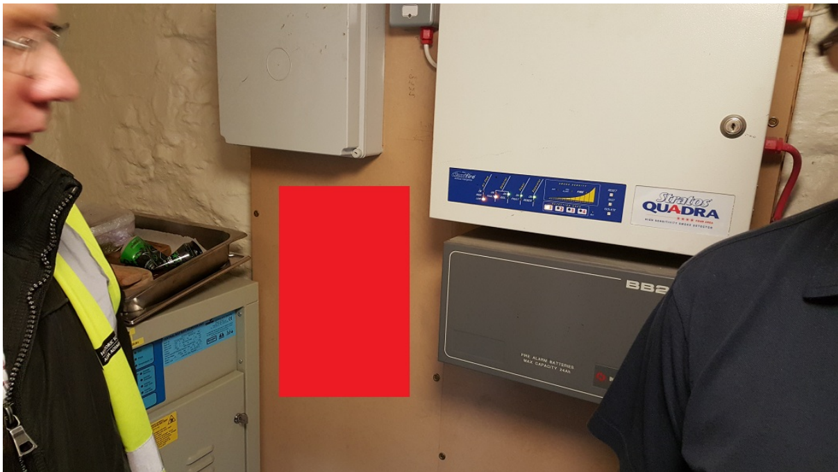
Fig. 8 Edinburgh Castle Gatehouse proposed Ethernet switch location, to be mounted on existing backboard
