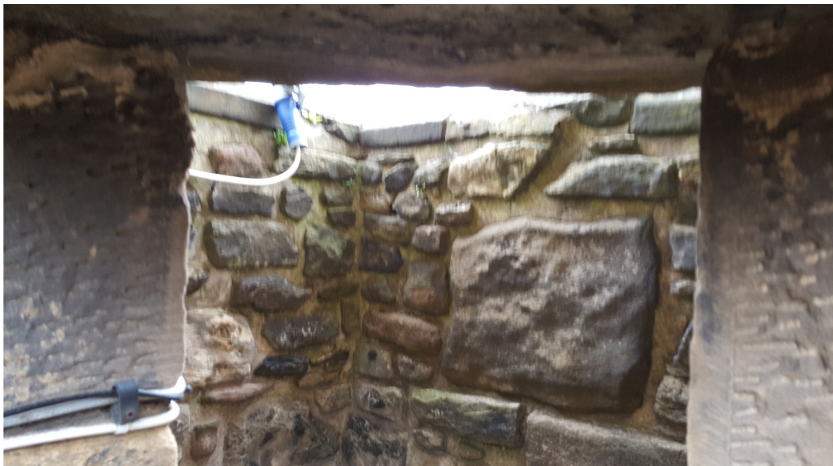
Fig. 14 AREA 3 - Edinburgh Castle Water Tank access point location – access point antenna will be pole mounted within this recess, positioned to be invisible from Hawk Hill, but in line of sight to New Barracks roof
